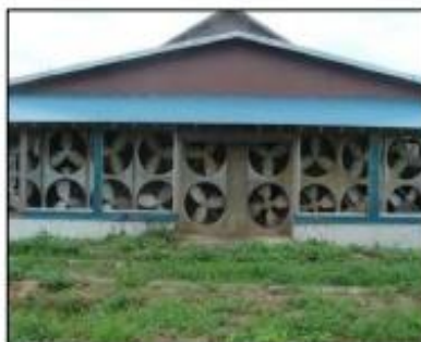
↑牛舎壁面の換気扇
